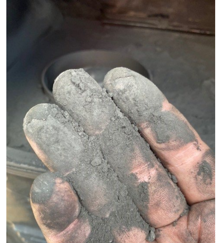
Dust deposited inside duct work of AC system
